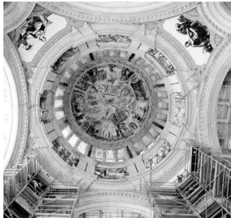
The current condition of the inside of the dome at Mnac building
