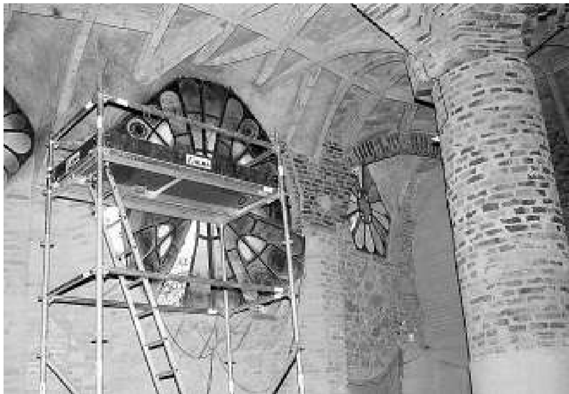
An exterior and interior view of the crypt at the Güell textile estate after public works were under way
