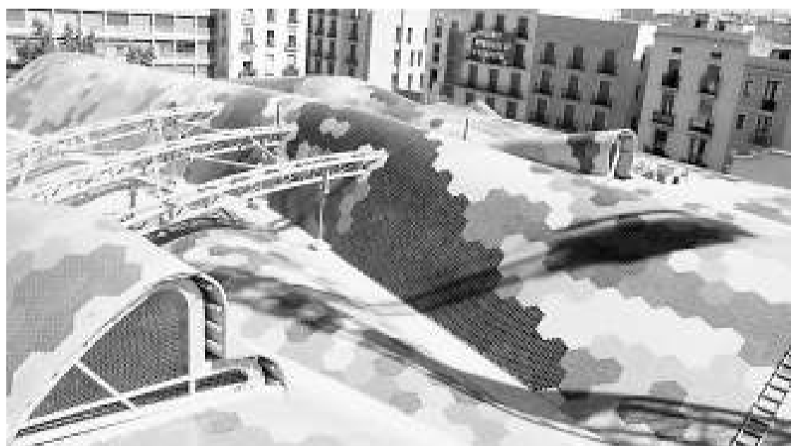
The remodeled market of Santa Caterina in the Barri San Pere in Barcelona which is due to reopen later this year
